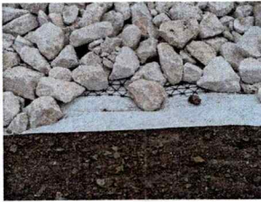
Coarse angular stone laid onto a geogrid and geotextile. Image from wikimedia commons
